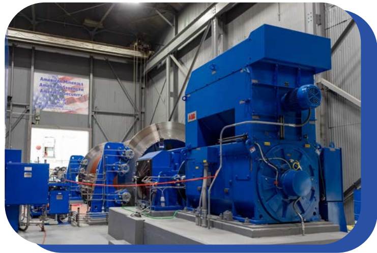
Jewell Shaft Hoist Room
