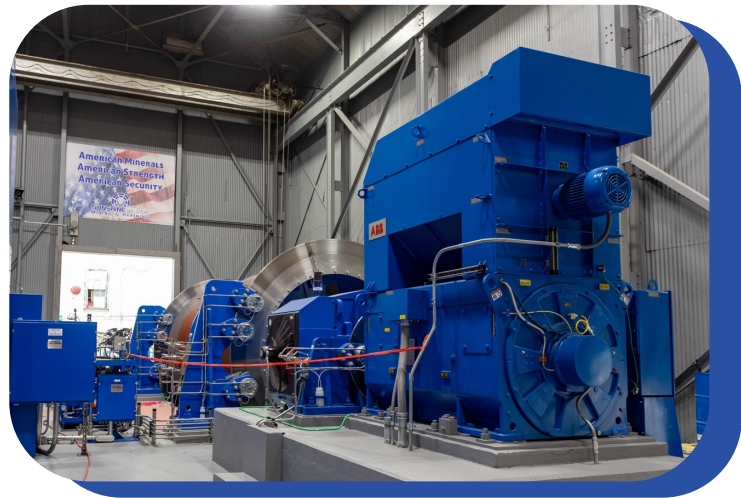
Jewell Shaft Hoist Room
